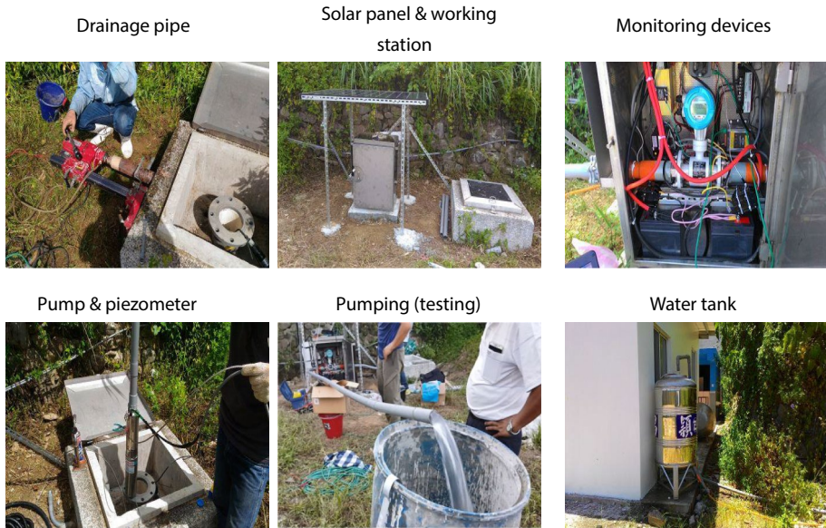
Fig. 14 Various components of the intelligent hazard prevention system installed and tested at the landslide site
